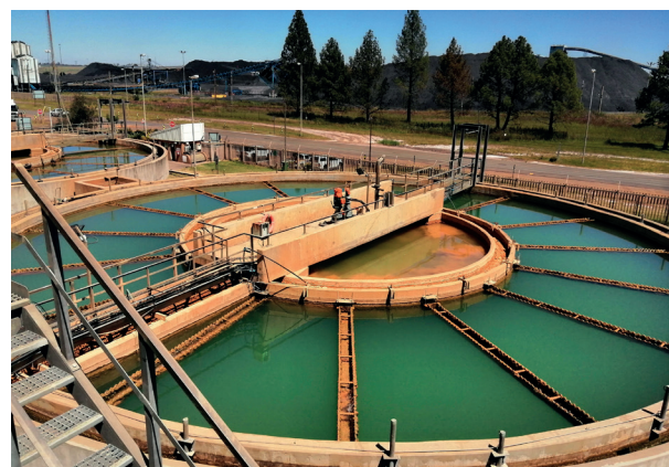
Mine water is fed into a sedimentation tank where it is treated.
